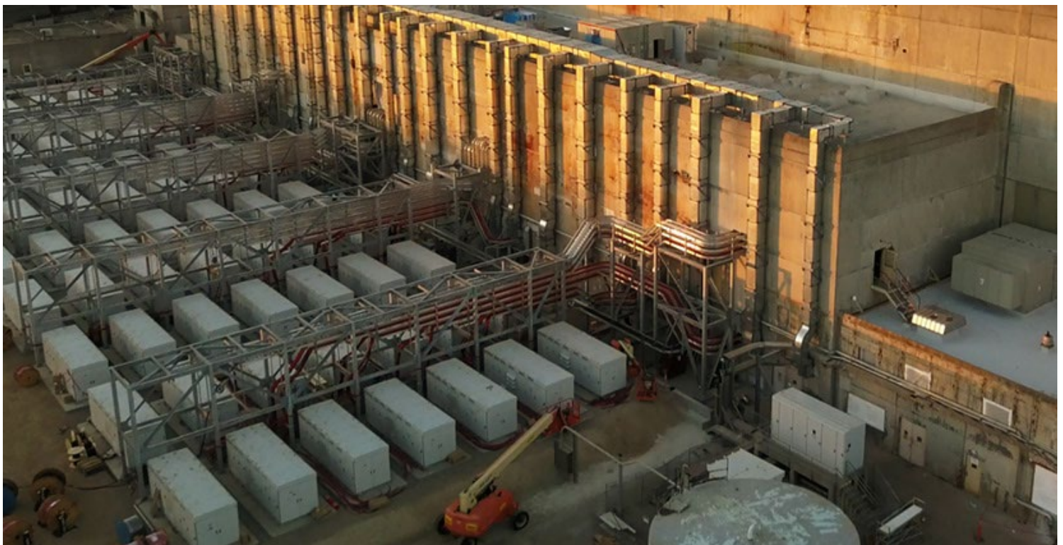
Vistra's Moss Landing battery storage project in California | Vistra
